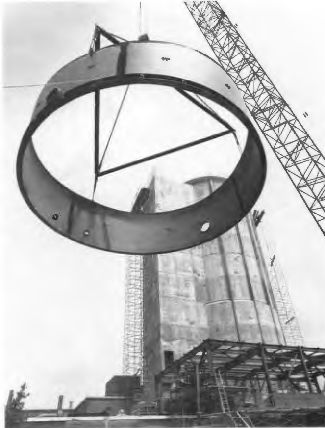
A crane hoists a ring to the top of the Holifield Heavy Ion Research Facility under construction during the 1970s.
