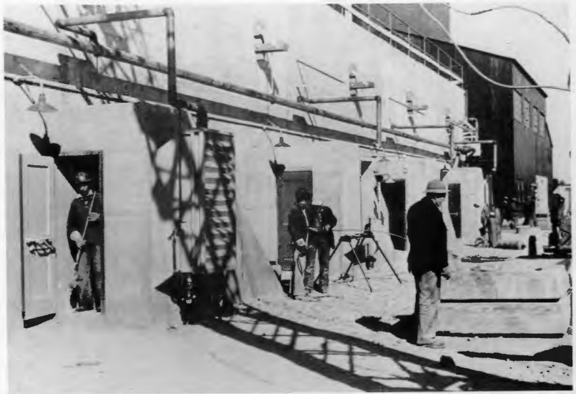
Constructing the concrete hot cells of the chemical separations building in November 1943. In 1992, this Radiochemical Development Facility (Building 3019) was designated a Nuclear Historic Landmark by the American Nuclear Society.
