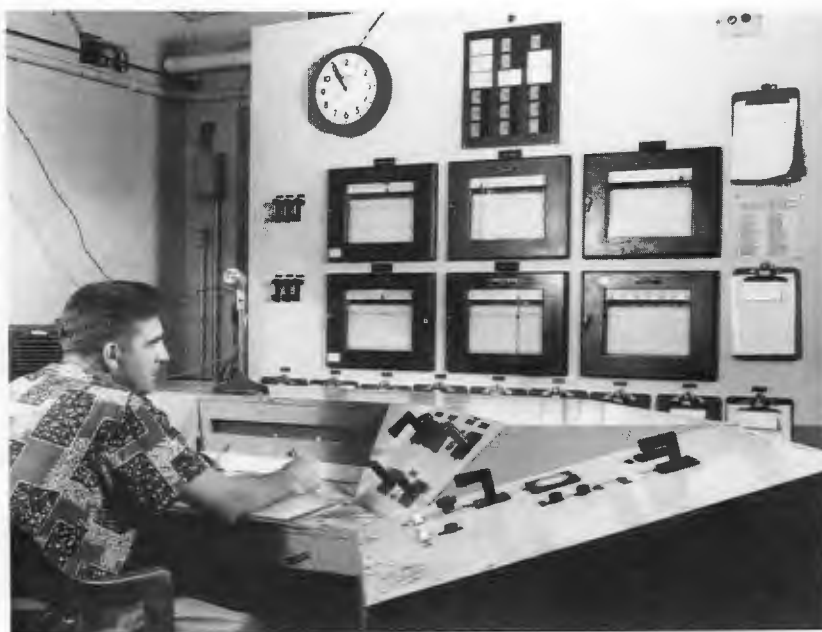
Control panel for the Low Intensity Test Reactor, built initially as a mock-up of the Materials Testing Reactor, which was designed in Oak Ridge and built in Idaho.
