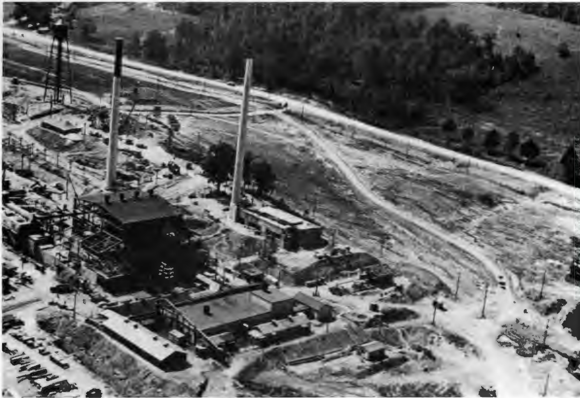
Clinton Laboratories, X-10 site, including the Graphite Reactor, under construction in October 1943.
