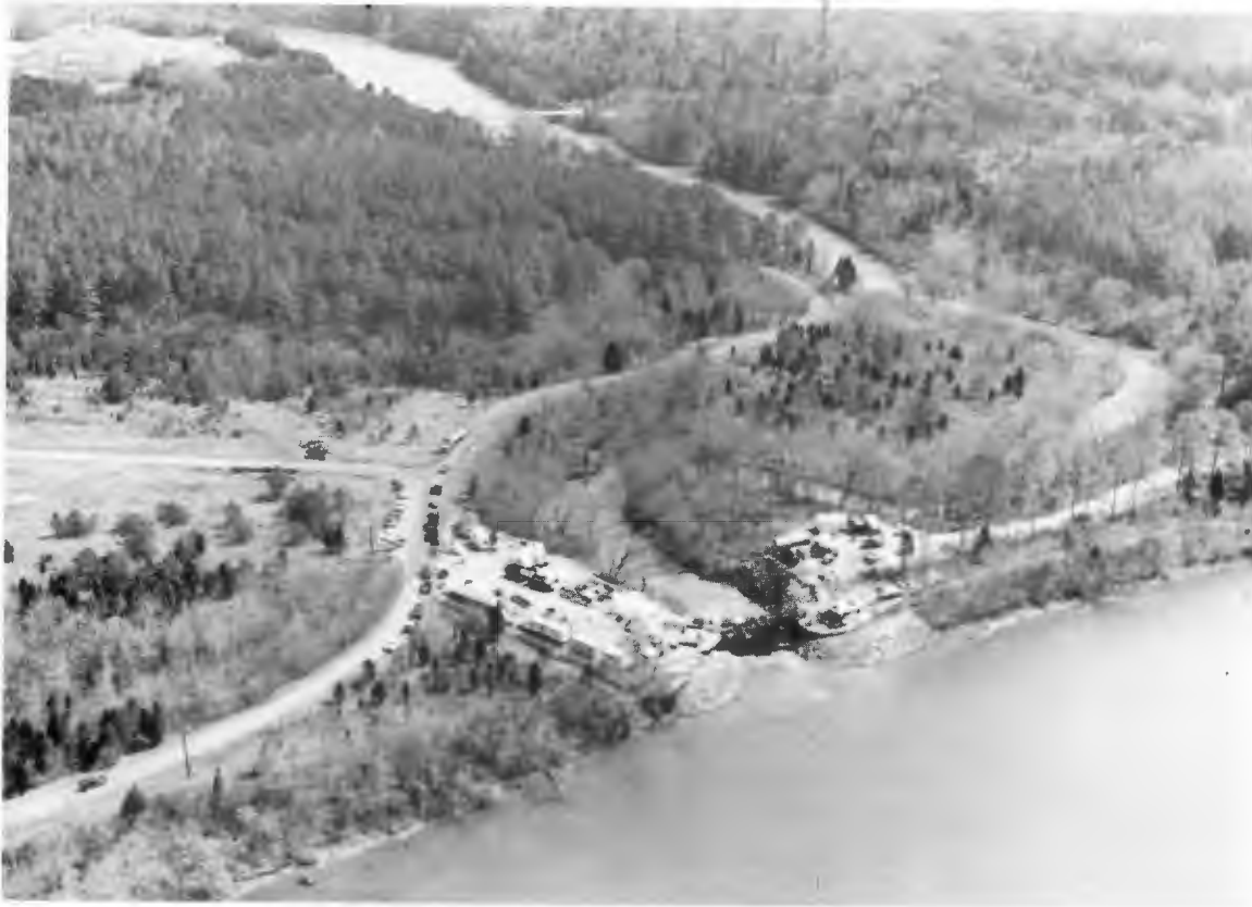
The White Oak Creek Embayment Sediment Retention Structure was built to stop releases of radioactive contaminants into the Clinch River.
